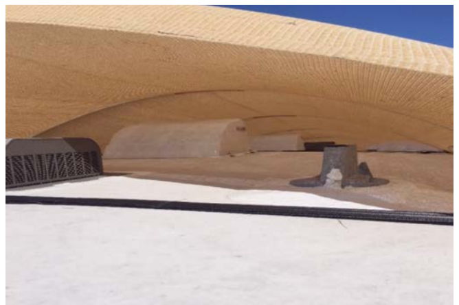
36) Notice roof unit clearance in front of RV.
