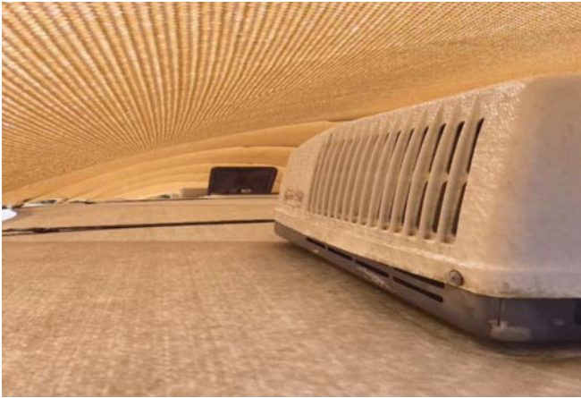
37) Notice roof unit clearance in back of RV.
